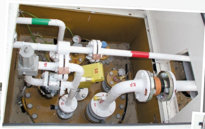
Underground autogas installation using one autogas series pump with one tank.
